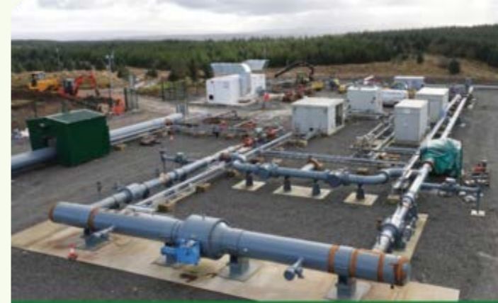
The £12.7 million HyNTS FutureGrid NIC project at DNV’s Spadeadam Test and Research Centre
